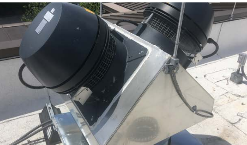
The RS16 Chimney fans and Powerstack EPS-1 system
